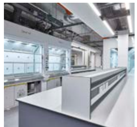
Innovative uses of cable trunking
