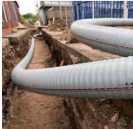
District heating & heat networks
