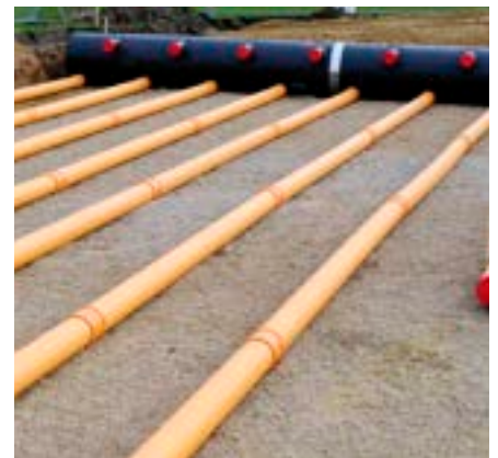
Ground-air heat exchanger
