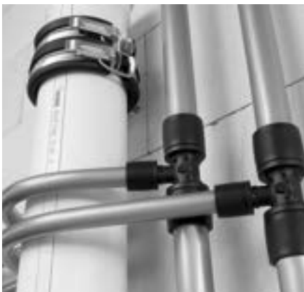
Polymer pipe for heating & plumbing
